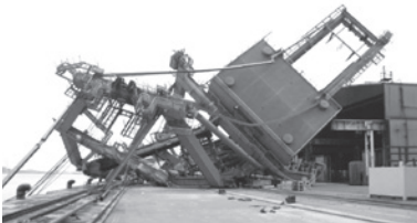
Damage to the wharf caused by a wrecked ship
